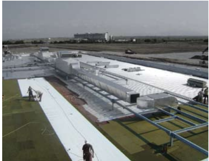
Construction of a steel roof with polymer waterproofing membrane on FIBRANgeo BP 70
